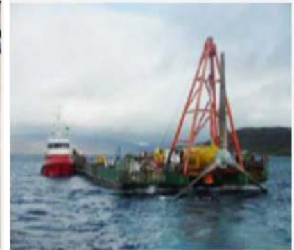
(f) Tidal Stream Turbine
